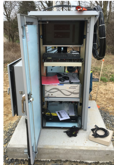
DiTeSt dedicated instrumentation cabinet
